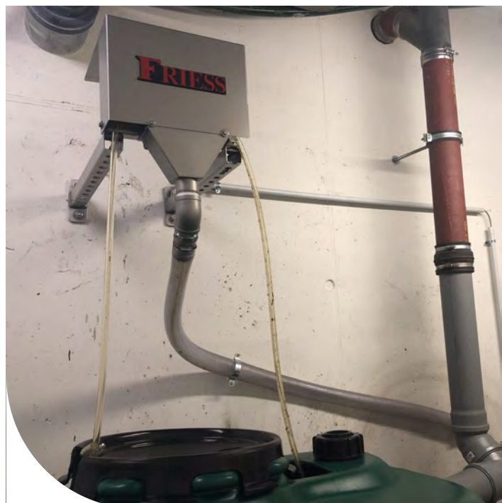
Oil skimmer in operation
