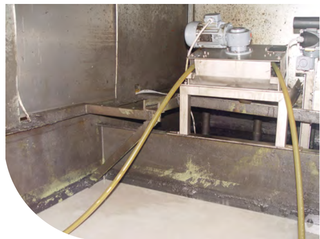
Oil skimmer in operation
