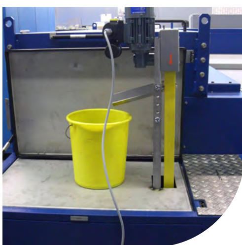
Oil skimmer BS at degreasing plant
